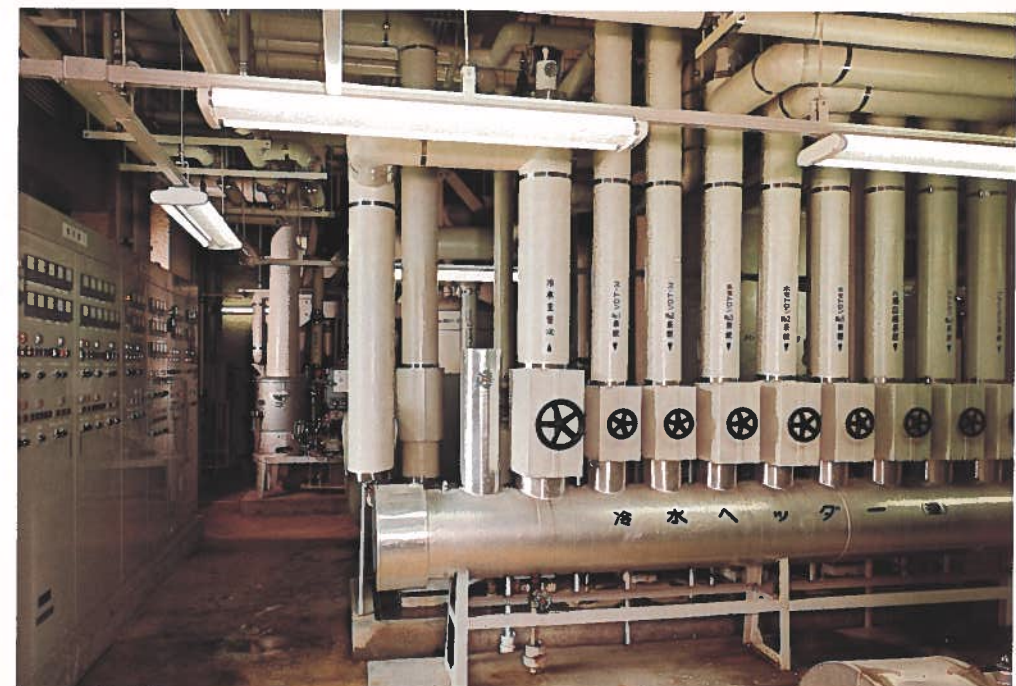
Fig. 2. Inside view of machinery room
