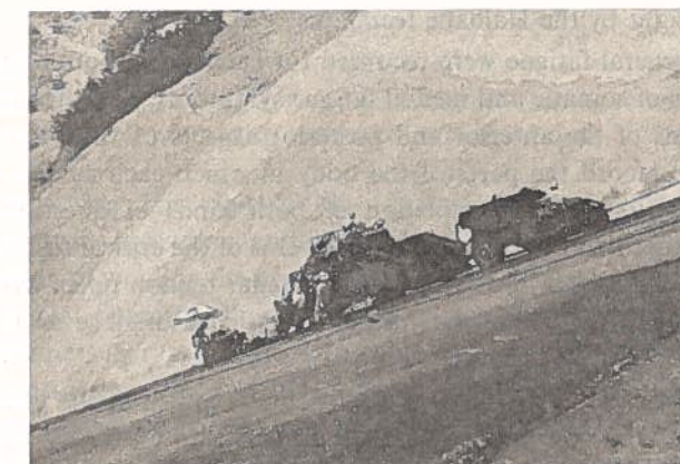
Fig. 1. Asphalt paving machines and workers on the slope of a rock-filled dam. From right to left, the dumper, the finisher, and the vibrating roller.
