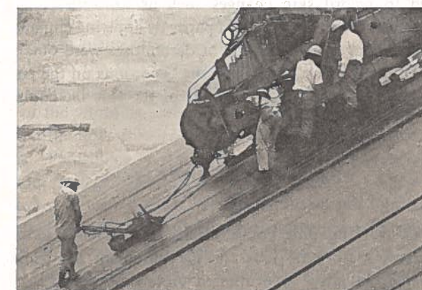
Fig. 2. Working postures of the standing workers on the slope surface. From right to left, two workers adjusting the finisher, a raking worker, and a worker manipulating a joint-compacter.
